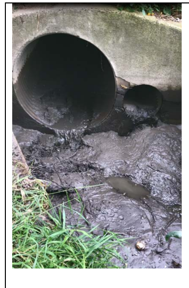
Screen shot of the city provided a video showing of sediment/mud flowing out of the culvert at Frontier Trail.
