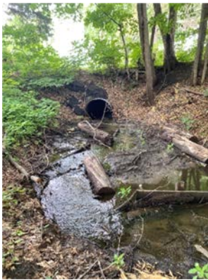
A. Sediment Accumulation in Ravine and storm sewer at Frontier Trail
