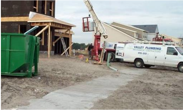
The process of suburban construction disturbs and compacts soils resulting in increased runoff and decreased stormwater infiltration.
